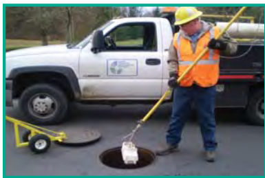
District Maintenance Specialist checking the status of a flow monitor in the District's service area
